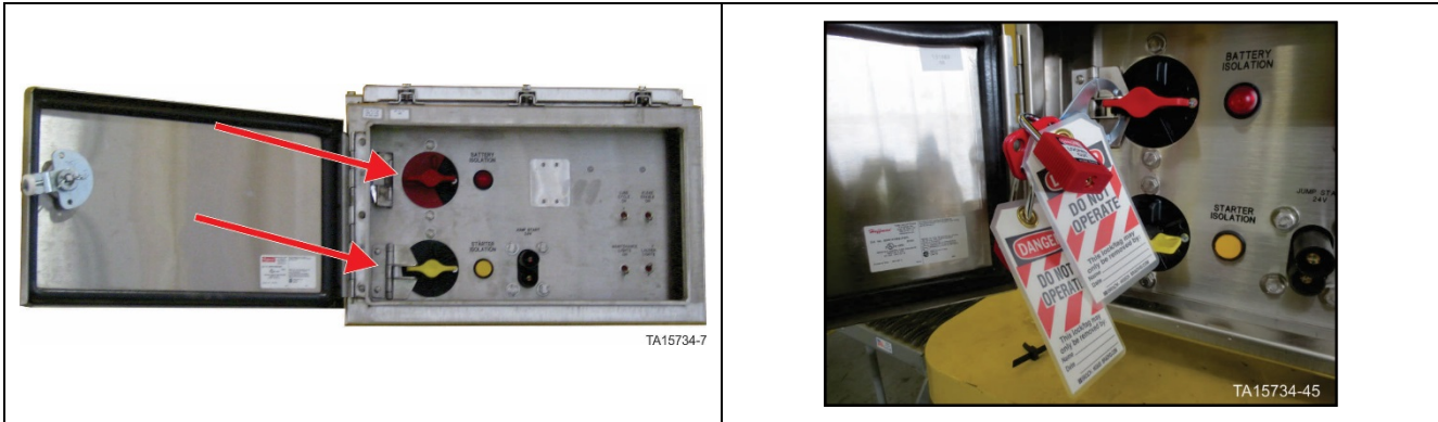
Figure 46. Battery Isolation Box – Battery isolation switch in OFF position with locks in place
