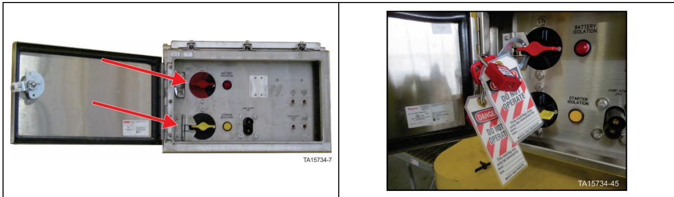
Figure 12. Battery Isolation Box – Battery isolation switch in OFF position with locks in place
